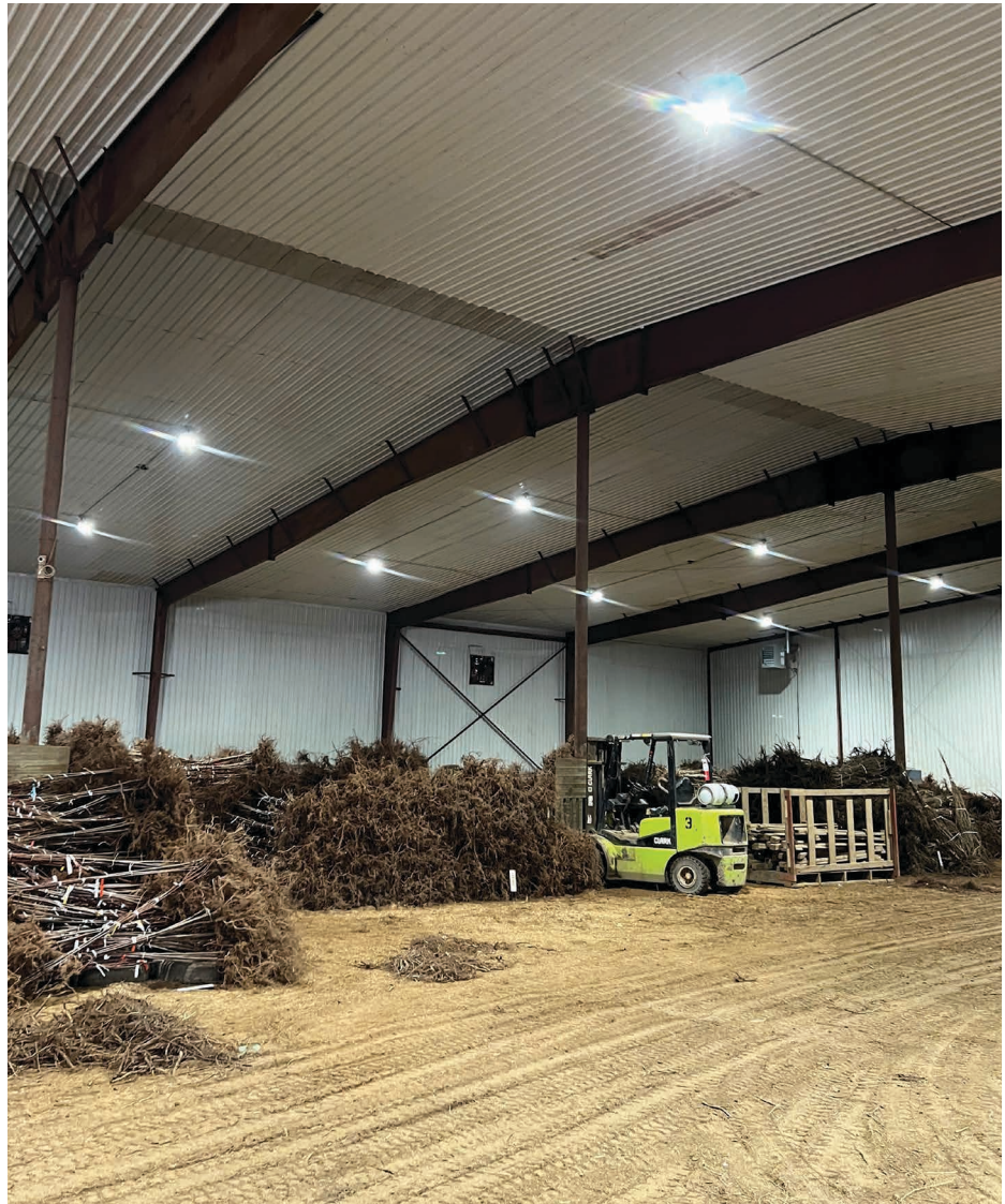
At Surface Nursery, high-bay sodium and mercury-halide lights were replaced with UFO-style LED lights. Every incandescent and fluorescent bulb at the nursery was replaced with LED, said Vice President Shawn Nerison. PHOTO BY SHAWN NERISON
