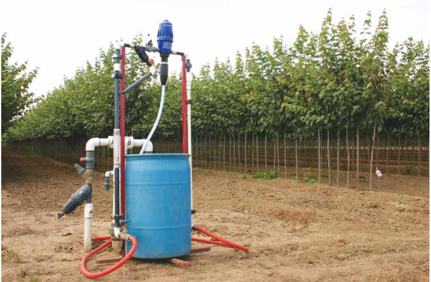
A fertilizer injection station and subsurface drip irrigation system manifold are pictured at J. Frank Schmidt & Son Co. The nursery applies liquid fertilizer through the system. PHOTO COURTESY J. FRANK SCHMIDT & SON CO.
