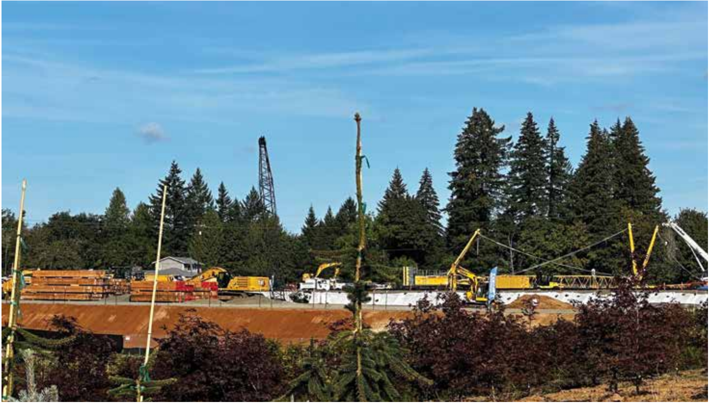
Construction at the site of the Portland Water Beaurau's filtration plant in East Multnomah County. PHOTO BY VIC PANICHKUL
