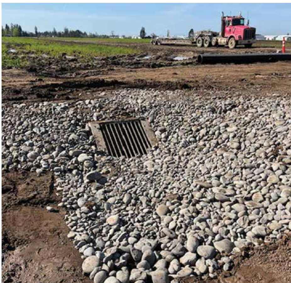
Designing a field for water drainage in the first place can help mitigate problems later on. PHOTO COURTESY OF HOSTETLER FARM TILING LLC
